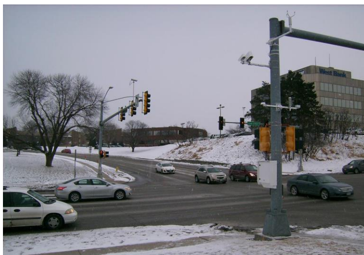
A fixed RWIS system installed on a West Des Moines street
