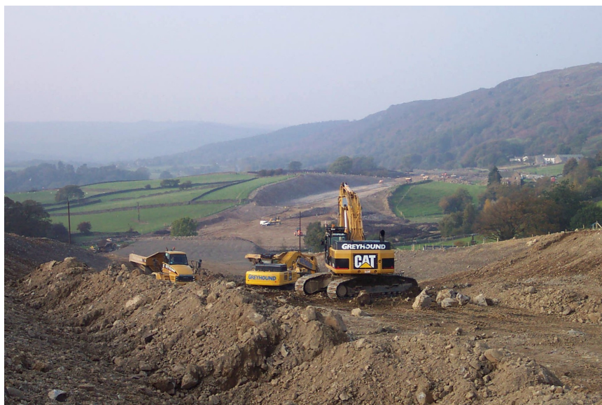
Above: 450,000m 3 of earthworks material were moved in just one summer period.
