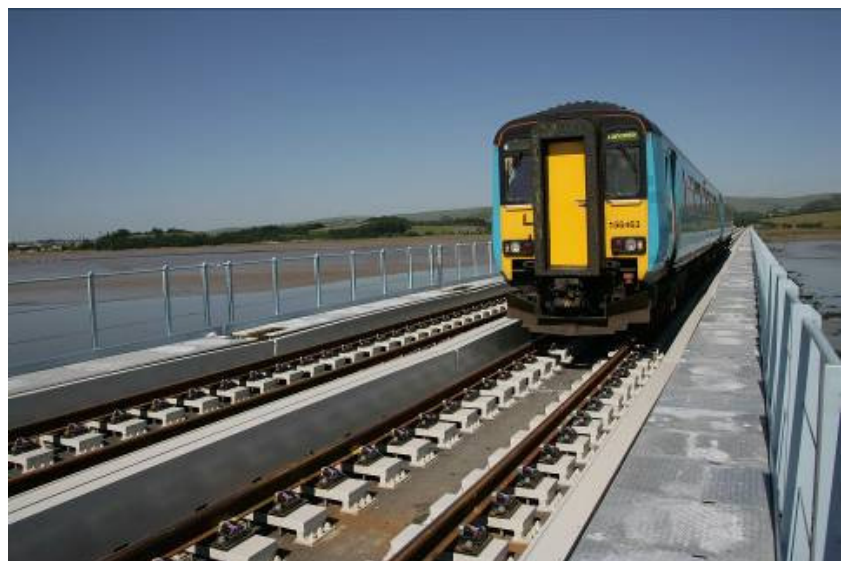
Centre Most works were undertaken from top down, to avoid disturbing the environment of Morecambe Bay
