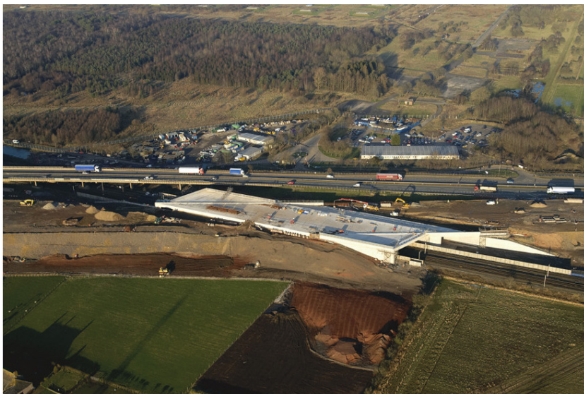
Above: Aerial view of the M6 Guards Mill Project, with the new Mossband Viaduct under construction.
