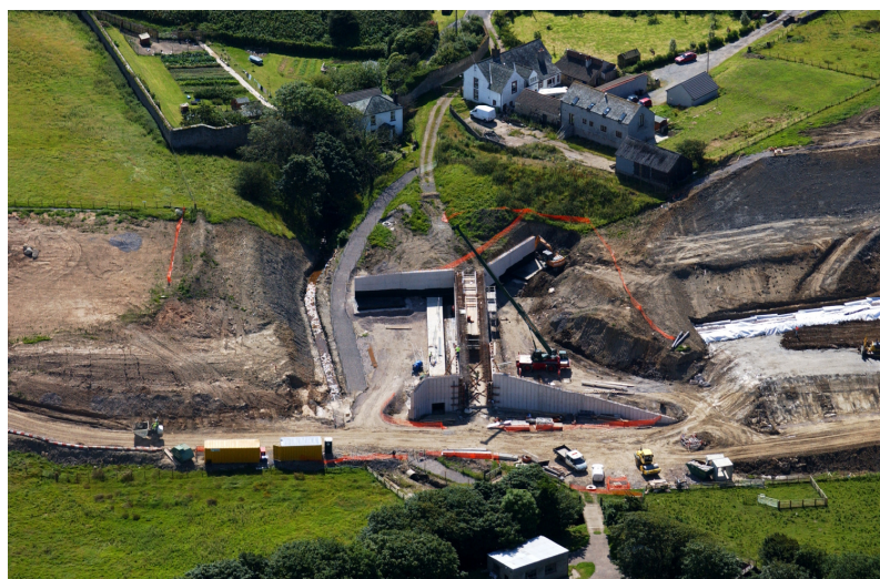
Top: Aerial view of A595 Parton to Lillyhall Improvement Centre: Lowca Beck Bridge Bottom: Ullgill Bridge
